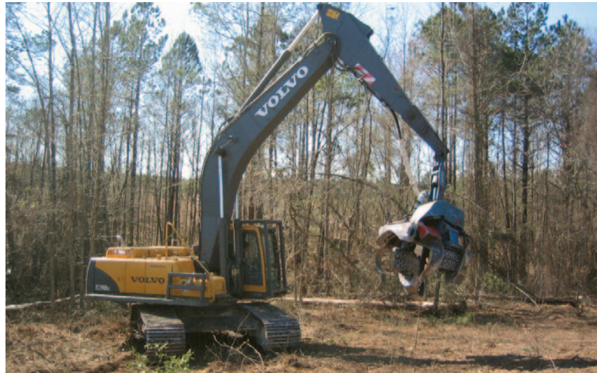
Ledbetter crews are using Volvo excavators to harvest timber more quickly and efficiently.
