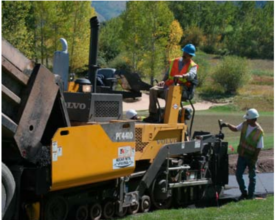
Ty Trulove of Glenwood Springs, Colo., started Rocky Mountain Paving in 2008 to handle smaller paving jobs.
