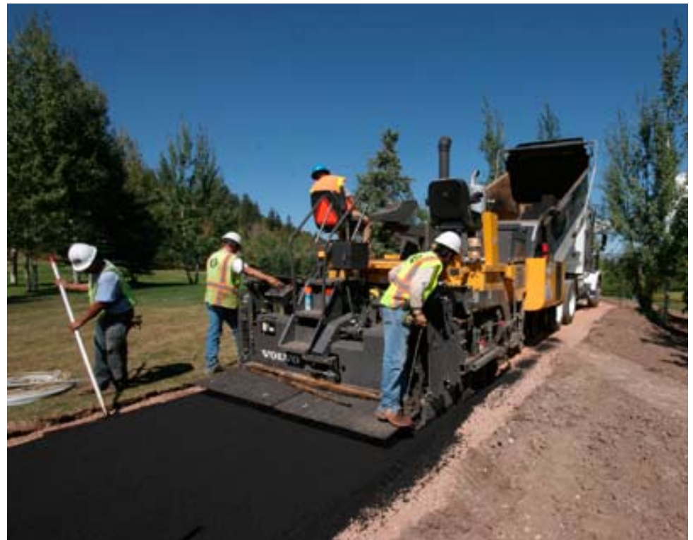
Adding asphalt paving services in addition to excavation gives Trulove a competitive edge.
