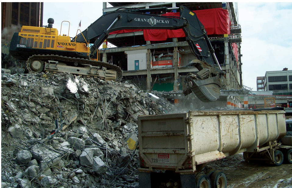
A Volvo EC700B makes easy work of the debris from the City Creek Center project in downtown Salt Lake.
