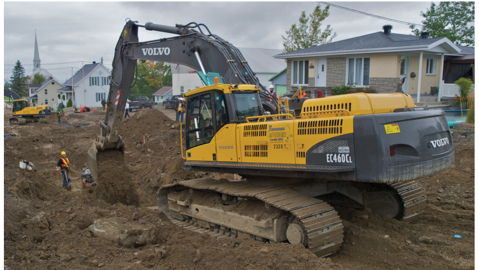
The historic eastern townships of Quebec are dotted with small municipalities, many with aging infrastructure. In Ste. Marguerite a Volvo EC460CL works in tandem with a Volvo EC210CL installing new sanitary sewers.
