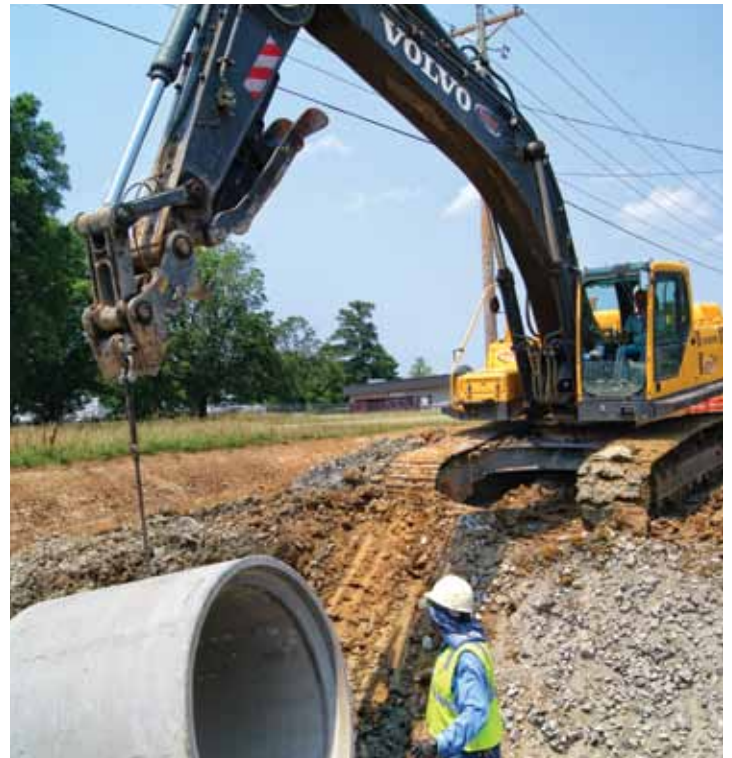
This Volvo EC360B easily maneuvers a 60-inch pipe into place during a street project near Little Rock.
