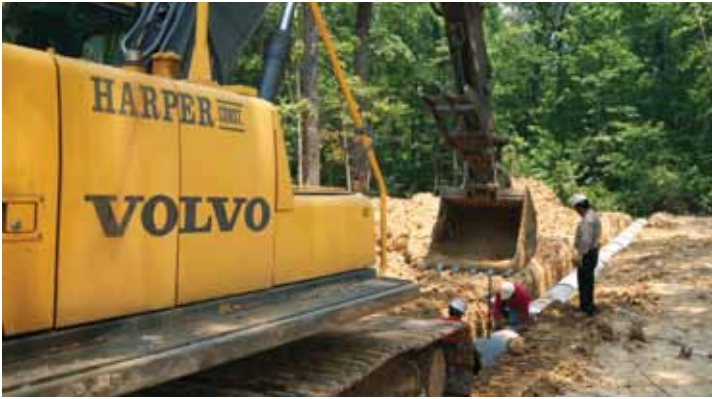
Digging trenches and laying pipe are par for the course for this Volvo EC210B excavator.
