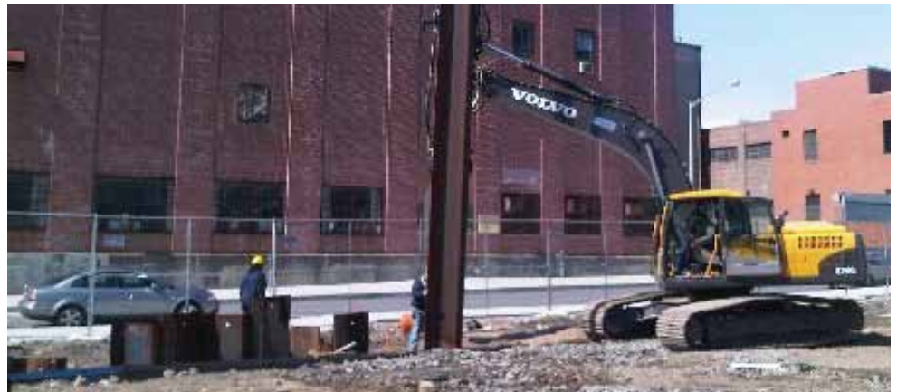
Frank T. Scobbo says the hydraulics of the Volvo EC240C deliver the drilling power needed to go 40 feet into the ground.
