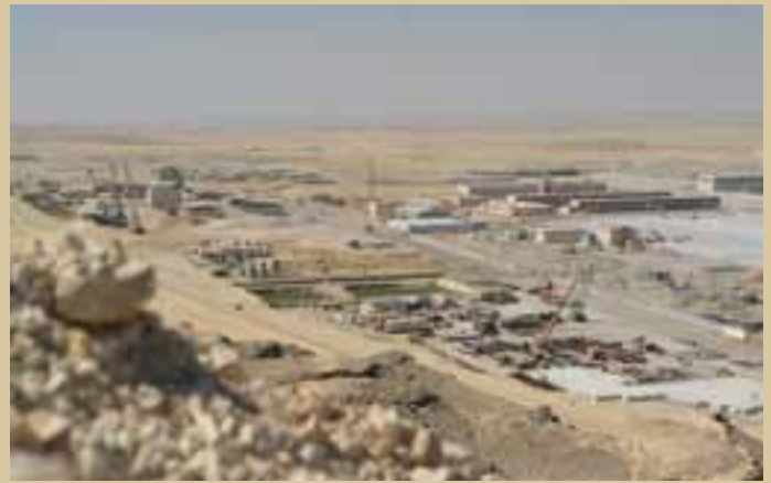
Duqm port - the biggest harbour construction project in the middle east today
