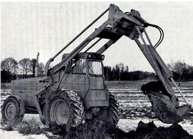
Narrow trenching for pipes or power cables, using a hydraulic excavator boom with 180° swing arc.
