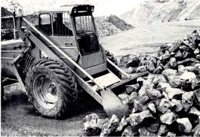
Mucking natural and blast quarry rubble, with sheet or open mucking scoop.
