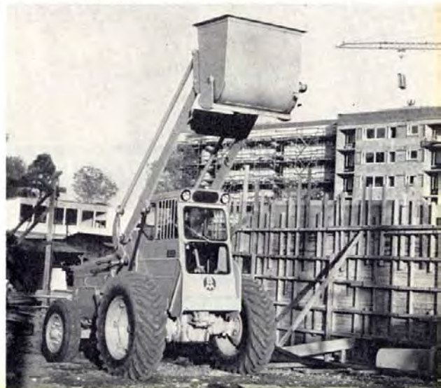
Transporting concrete, mortar and other bulk materials with the hydraulically-operated, bottom-dumping concrete bucket.
