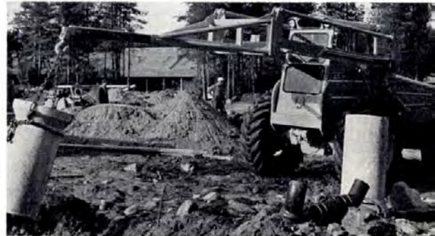
Pipelaying, materials handling and machine removals on construction sites, using the extendable crane jib.
