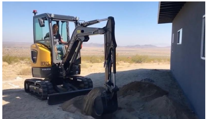
The ECR25 Electric performed various tasks in helping to build off-the-grid homes
