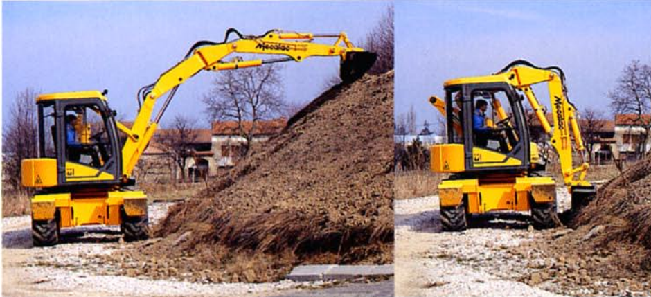
Creation of a 6 metre embankment down to the wheels without blocking the carriageway.
