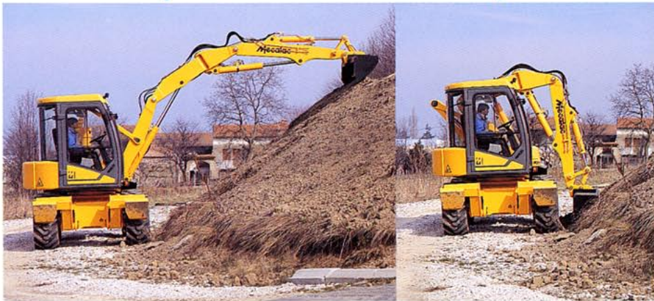
Creation of a 6 metre embankment down to the wheels without blocking the carriageway.
