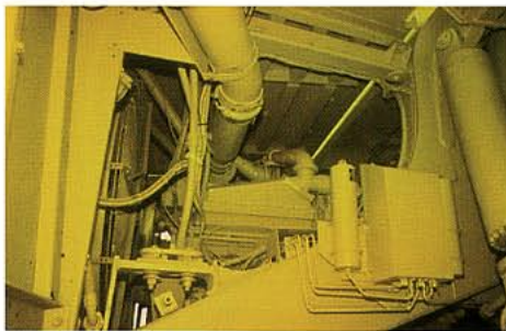
Ground level access to brake valve pack and test ports.
