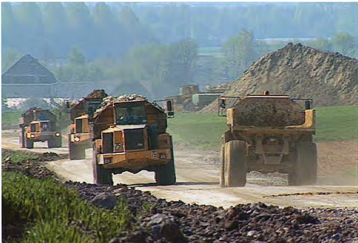
65 Volvo articulated haulers during the work of moving 2.5 million cubic metres of soil to prepare the way for the high-speed TGV train in southern Belgium.
