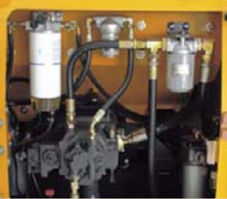
• Easy access to hydraulic pumps and filters.
