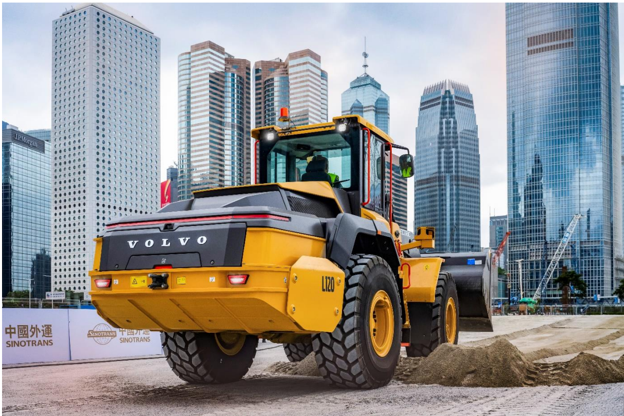
The new L120 Electric wheel loader is building and maintaining the racetrack in the heart of Hong Kong
